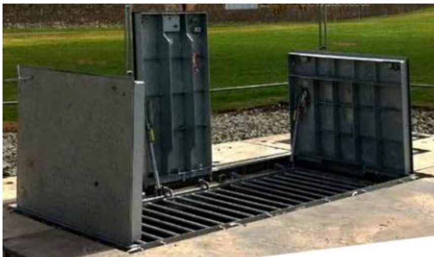
Figure 3-2 Surface Access covers
