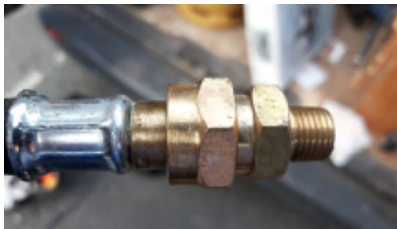
Photograph 7: Non return valves only
