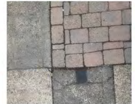
Poor and inconsistent paving materials
