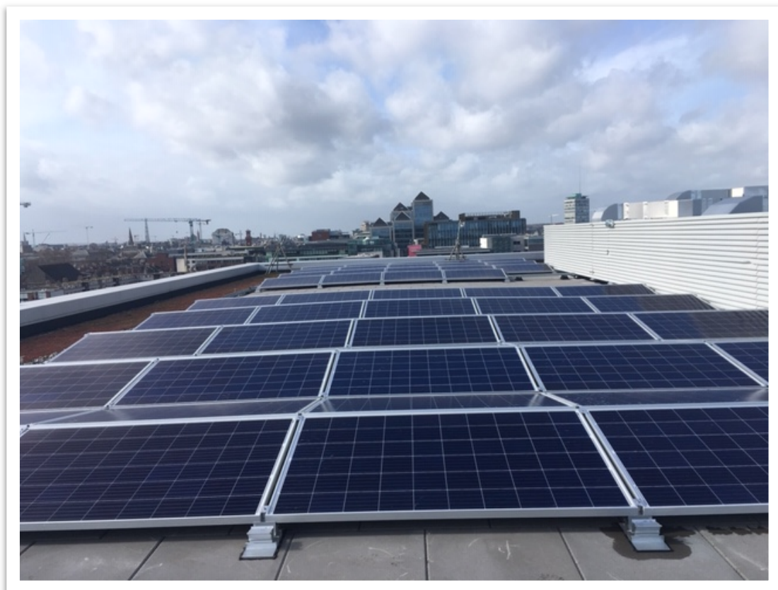
Figure 2: Typical PV array installation
