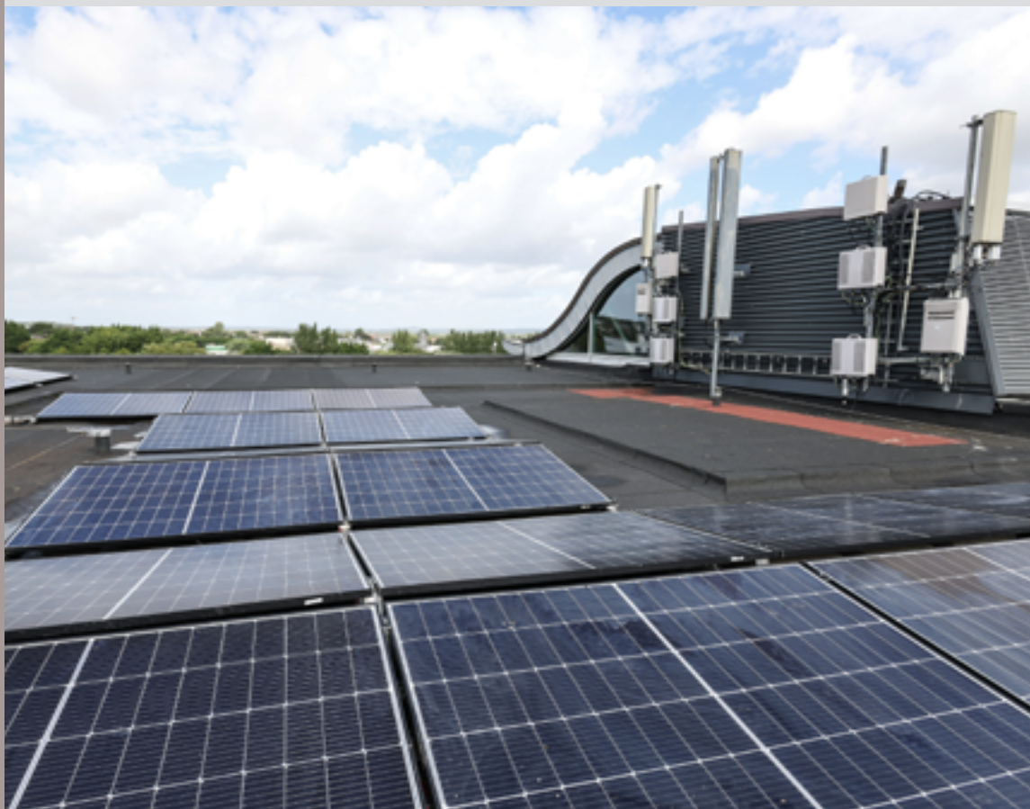
Solar PV installed on Fingal County Hall Rooftop
