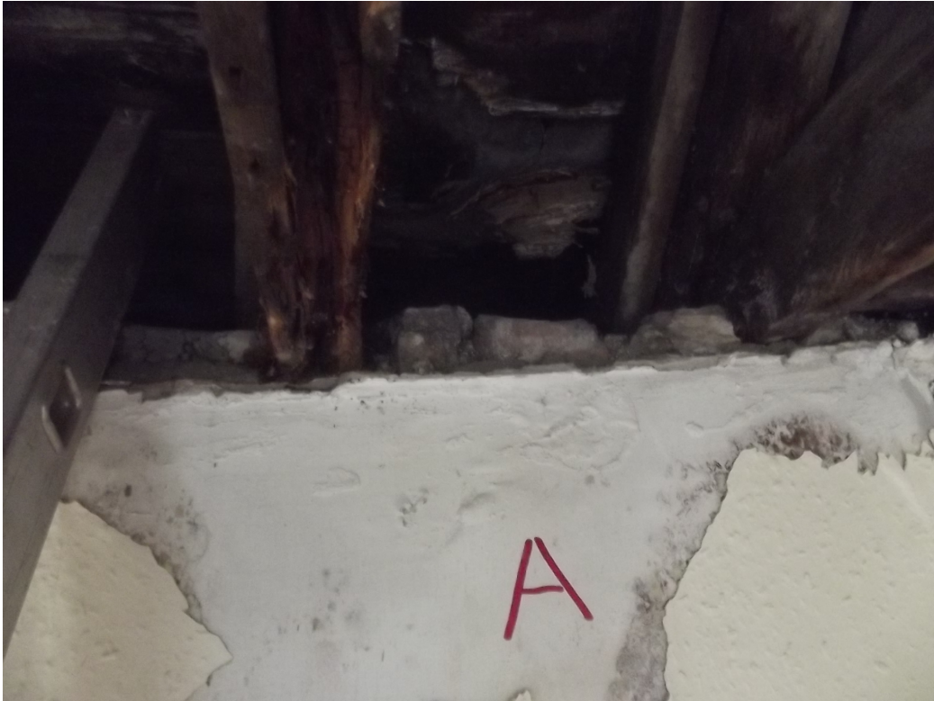
Figure 5. Decay at central valley. Severe decay to all components under lead valley.
