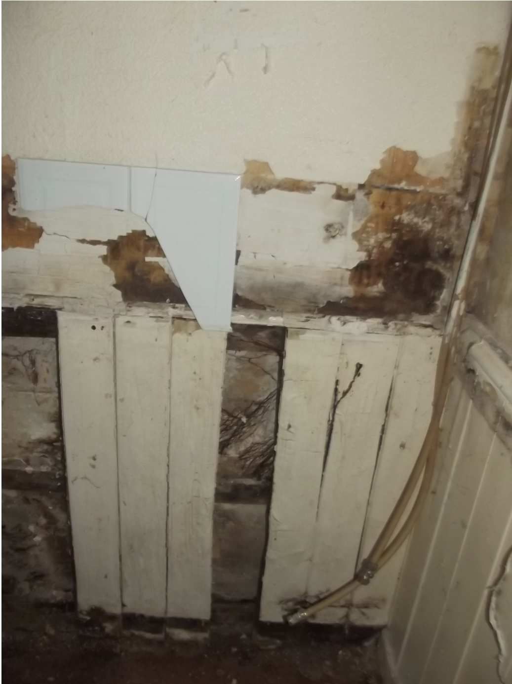
Figure 2. Decay to wainscoting in kitchen.
