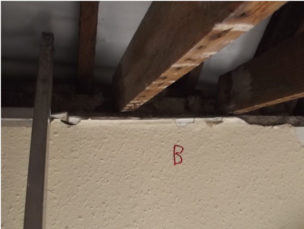
Figure 6. Rafters and ceiling joists on separate wallplates at front, not fixed together.
