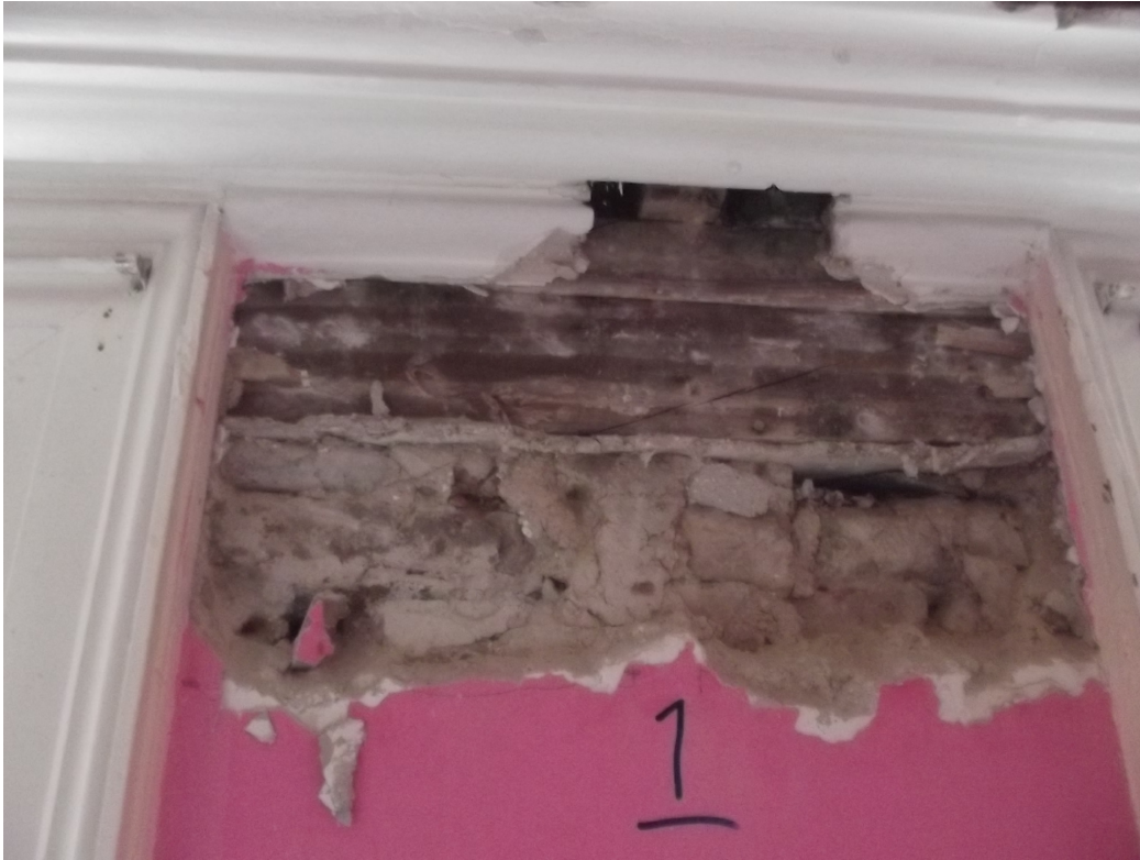
Figure 1. Heavy head across windows, living room northwest corner, with plaster to underside of head and marks of laths on face.
