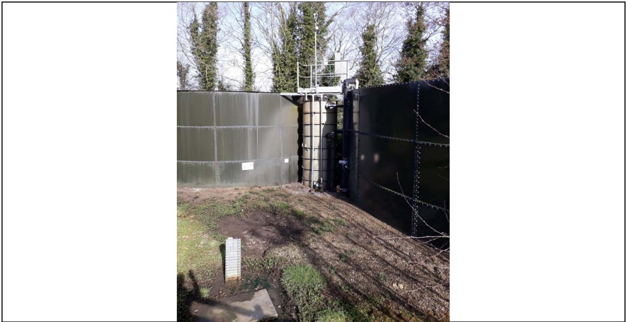
The SBR Unit and the Equalisation Unit
