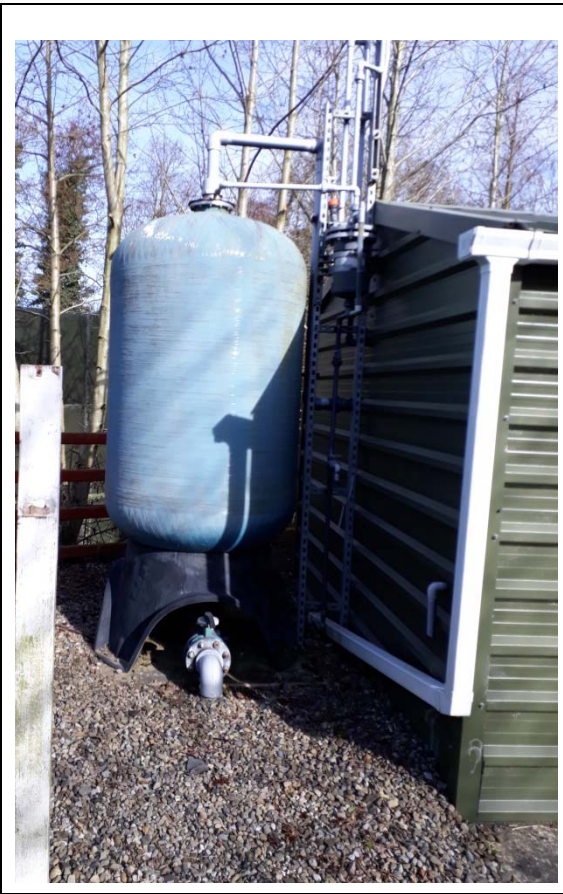
Ozone Reactor Vessel
