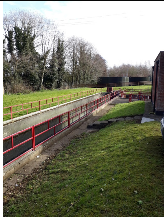
The existing oxidation ditch which is now used as a storm holding tank
