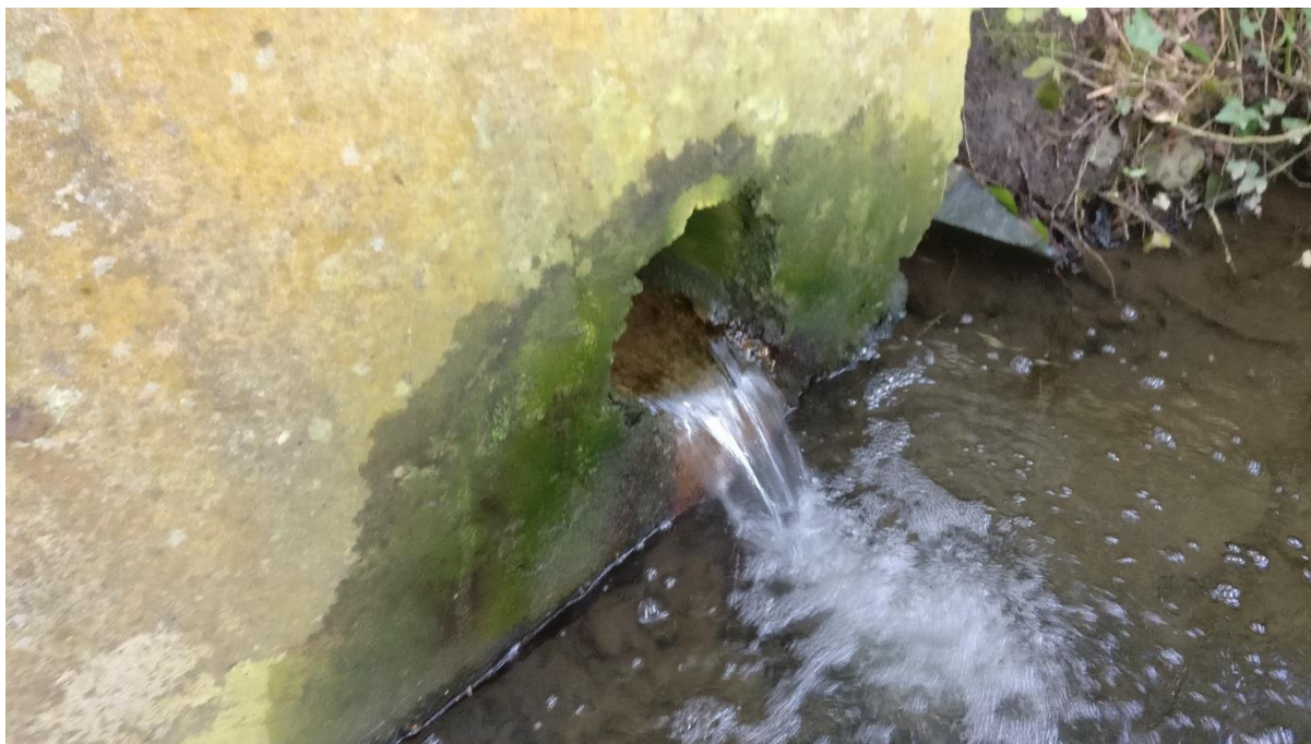
Figure 4-3: Primary discharge Garristown WWTP
