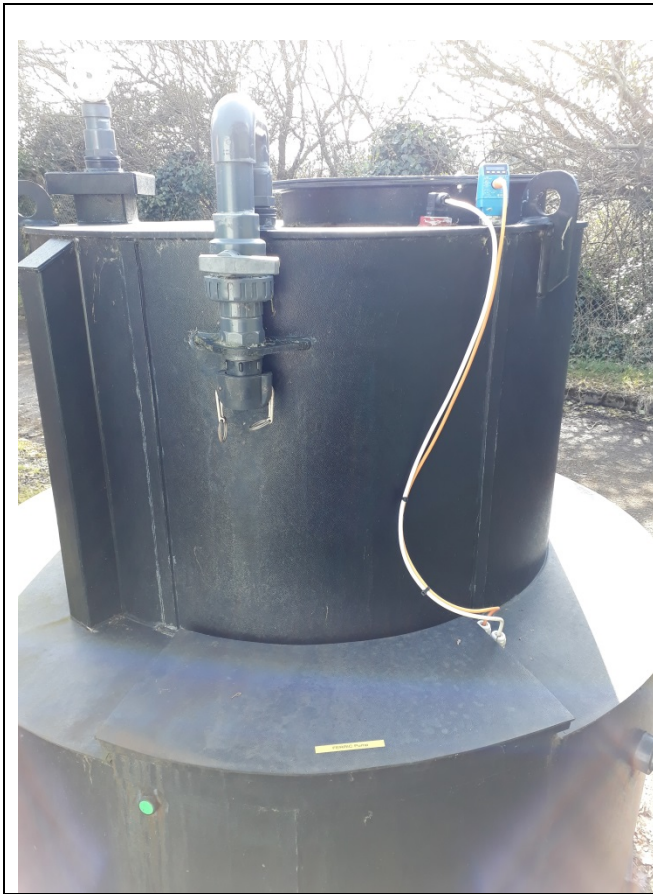
Ferric dosing unit
