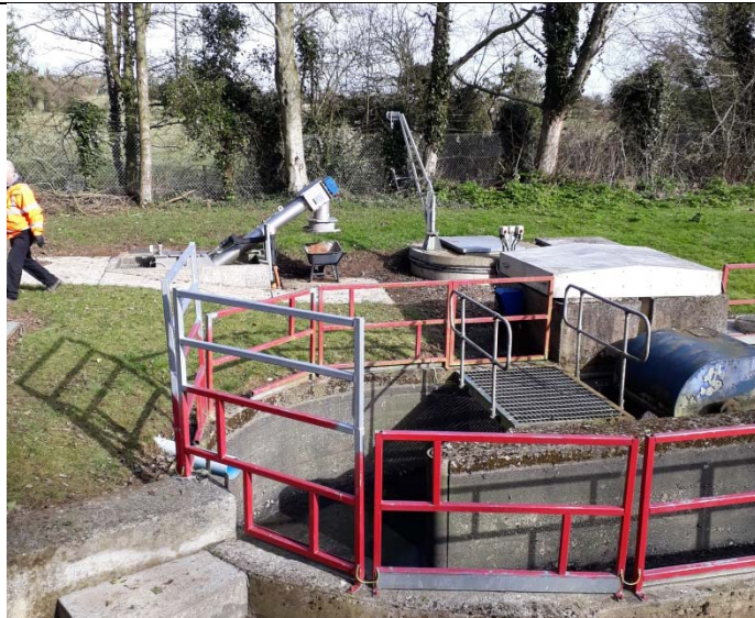
The inlet screen and the pump sump
