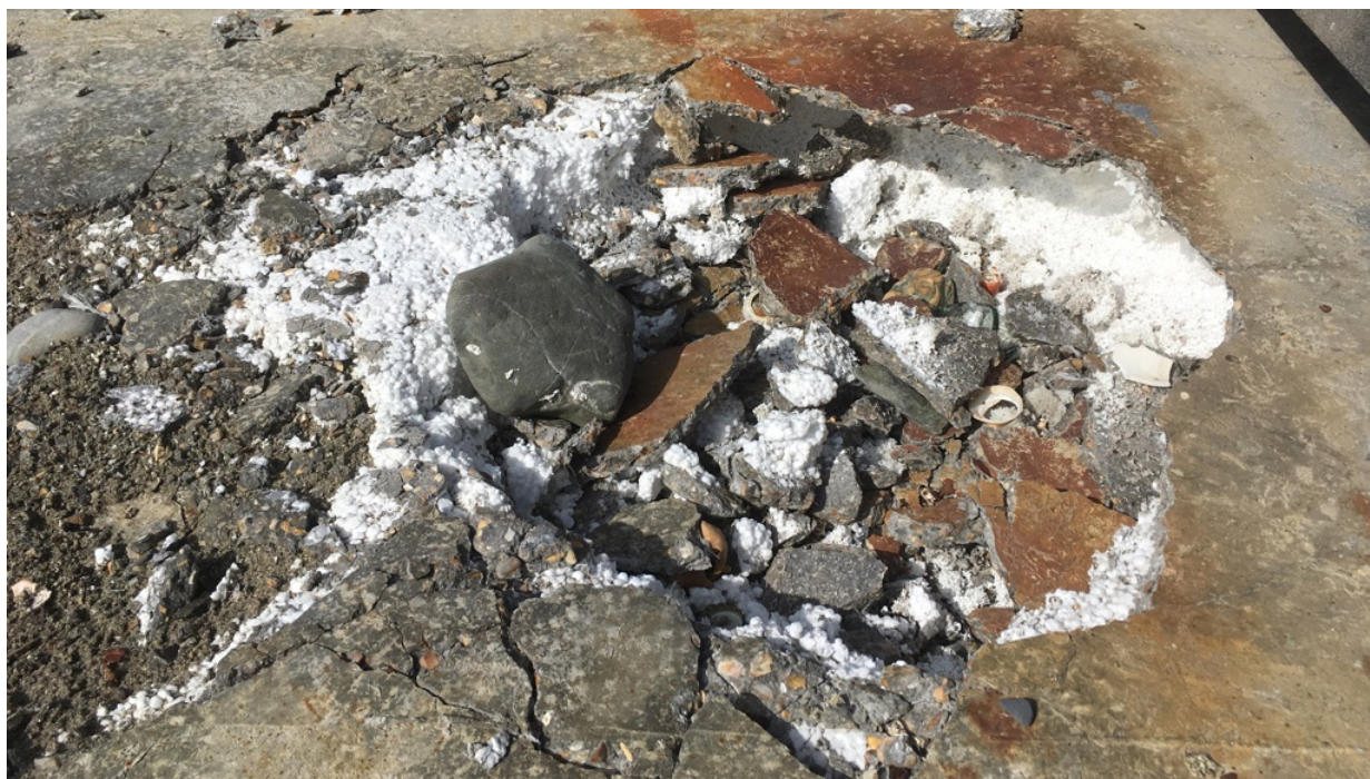
Figure 9: Erosion on the cement faced upper pontoon
