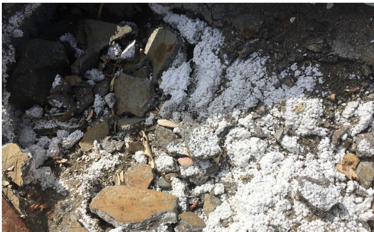
Figure 10: Eroded polystyrene core and exposed base of the pontoon
