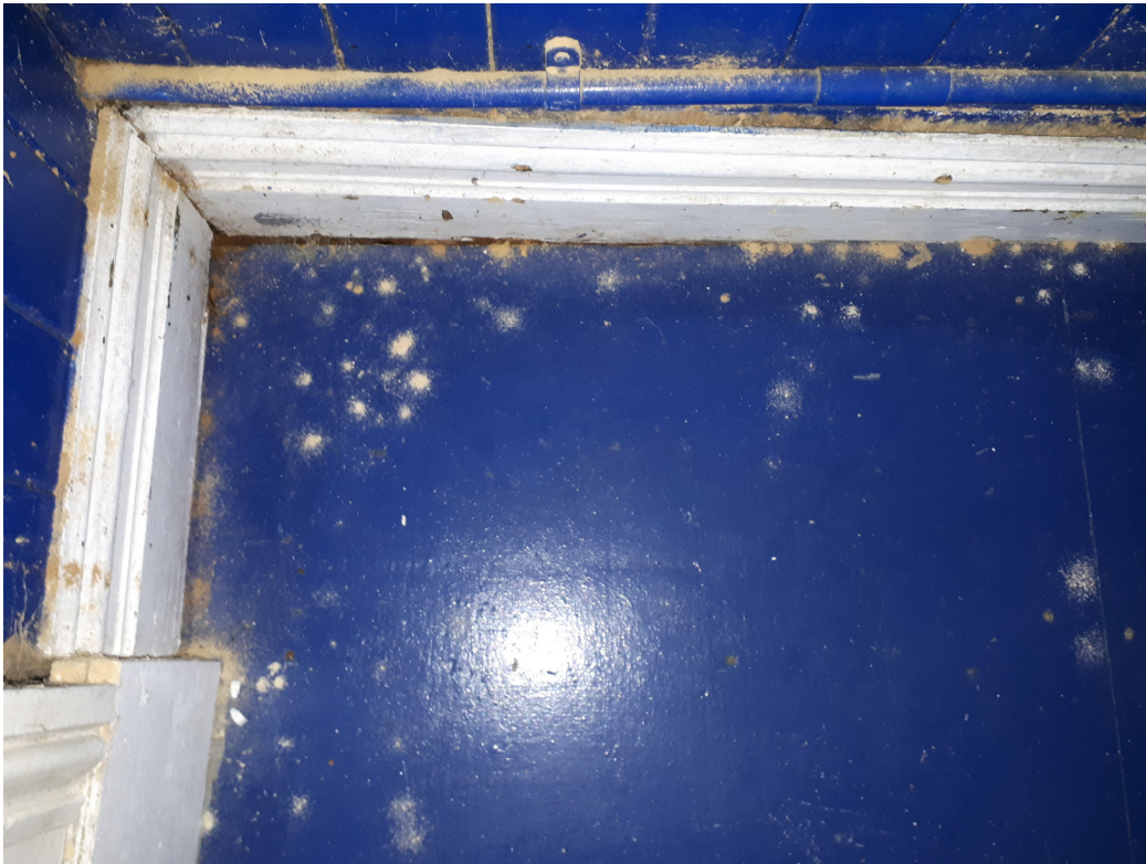
Figure 2. Severe insect attack, with piles of boredust from emerging adults.
