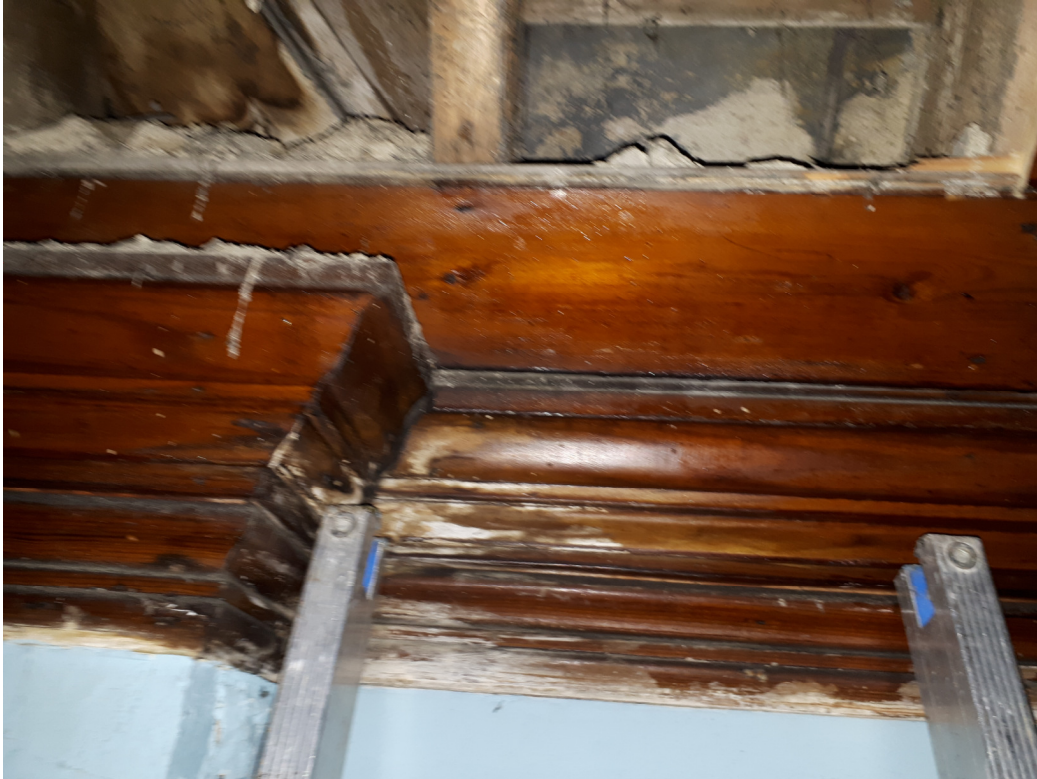
Figure 3. Water staining to cornice (bottom), and to valley board at top left.
