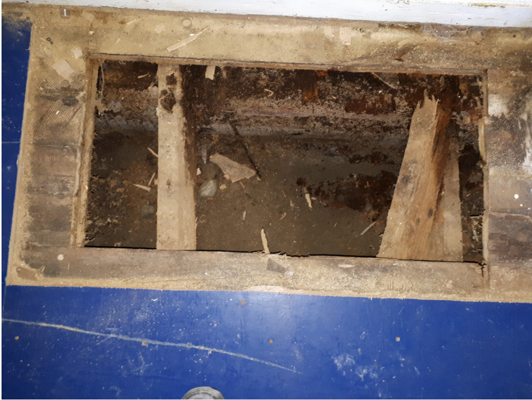
Figure 1. Severe decay to wallplate and joists, ground floor.
