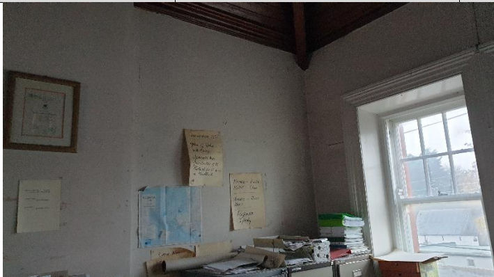
Figure 1 Damage to plaster at south gable wall due to water ingress from flat roof gutters
