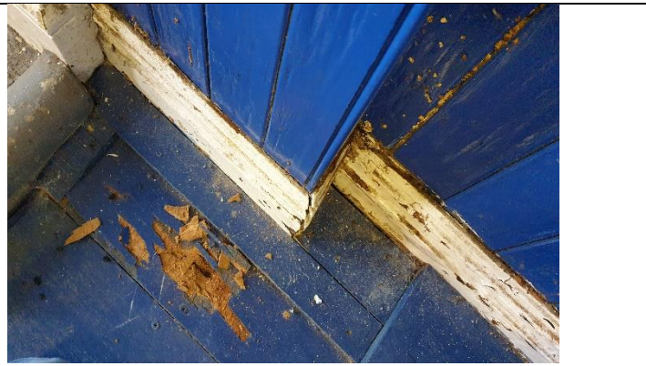
Figure 8 Decayed timber skirting and floor boards to RHS of fireplace
