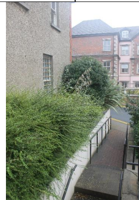
Figure 8 Soil and plant built up against east and north walls, possible source water ingress.
