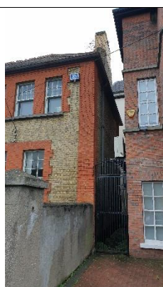
Figure 3 South elevation with buff coloured brick in an English Cross or Dutch Bond with alternating rows of headers and stretchers.
