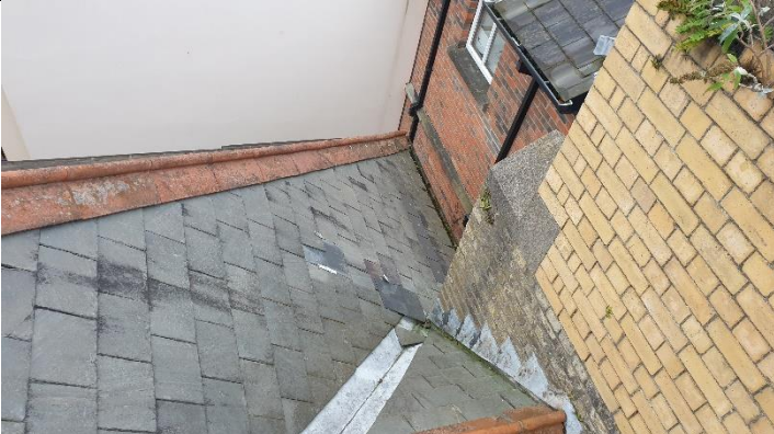
Figure 5 - View of roof from the south-east- Note slipped slates 1/3 down slope of roof
