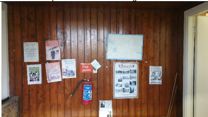
Figure 3 Full height TG+V varnished soft wood panelling to partition forming lobby – not original to building
