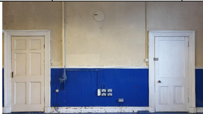
Figure 2 Evidence of timber decay at LHS of door to reception
