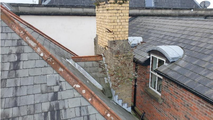
Figure 3 View of gusset roof with lead flashings at valley and abutment with chimney – change of colour of brickwork to upper section suggests chimney has been rebuilt or extended.
