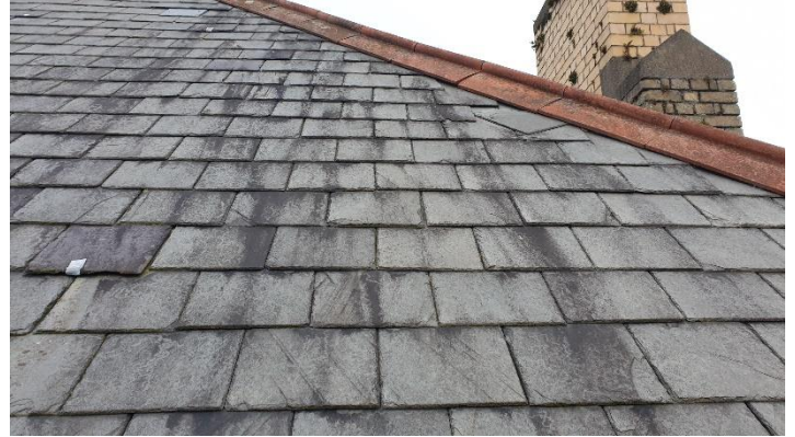
Figure 2 Close up view of north-east slope with further examples of recently slipped and previously repaired slates using lead strap hangers
