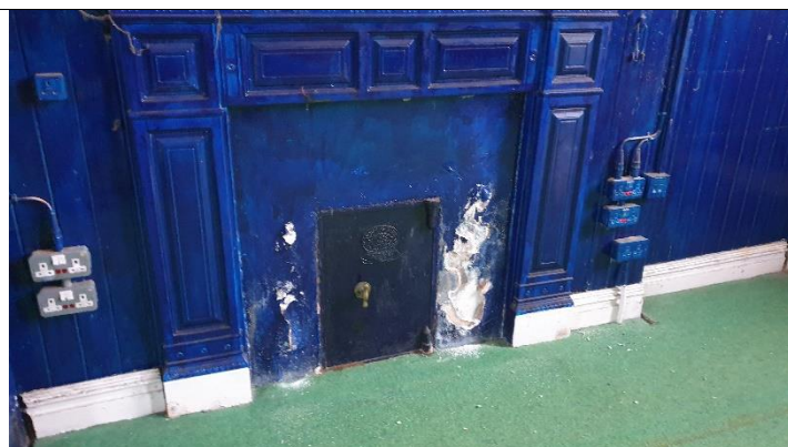
Figure 6 Fireplace surround at south wall (gable end) fire grate has been infilled with a metal safe- evidence of water ingress with in fire grate
