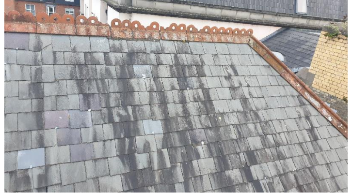
Figure 2- to right hand side of stairs out-crop Original natural slate roof with various sections of slipped and broken slate
