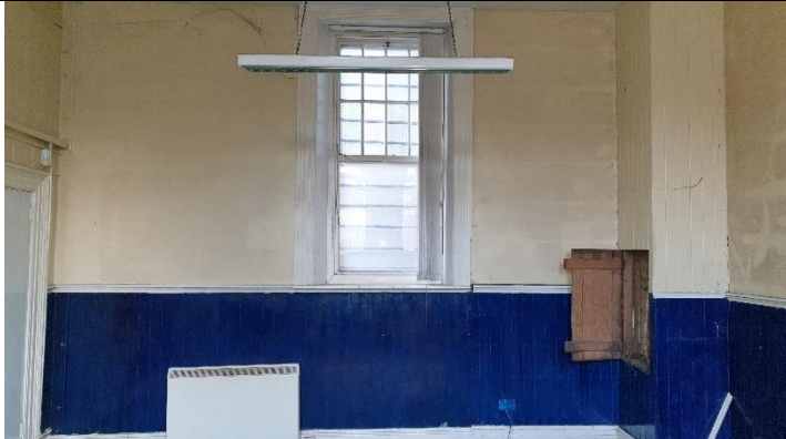
Figure 1 Evidence of timber decay – possibly dry-rot at junction with floor, between window and door.
