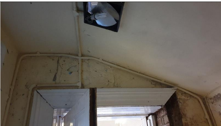
Figure 3 Boasted plaster at high level to RHS and LHS of window
