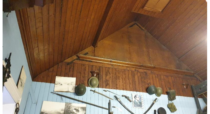
Figure 4 Section of wall within triangular roof truss area appears to be plywood sheeting infill – stained to
