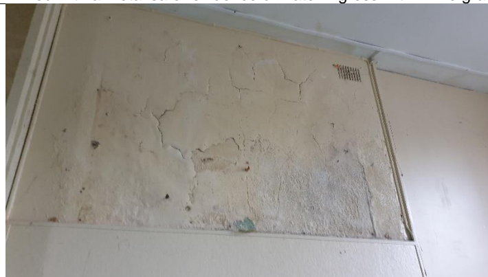
Figure 8 Severely boasted plaster at wall above fireplace, walls above dado on either side of fireplace is hardboard
