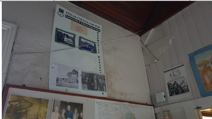
Figure 2 Severe damage to plaster at wall next to stairs due to water ingress from flat roof/parapet area
