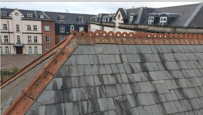
Figure 3- to left hand side of stairs out-crop Terracotta ridge and hips – ridge with decorative feature , hips with rolled top. Sections of ridge loose and in vulnerable condition.
