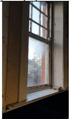
Figure 7 Windows to west - 9 over 1 single glazed sliding sash / painted soft wood – poor condition
