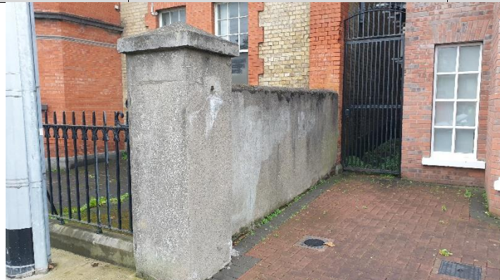
Figure 2 Gap between buildings is in ownership of adjacent building however eaves, gutters and rainwater pipes over sail.
