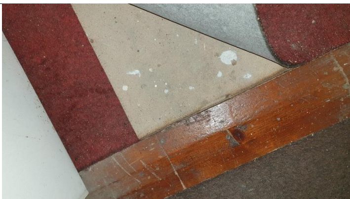
Figure 7 Carpet on plywood backing in poor condition- timber threshold
