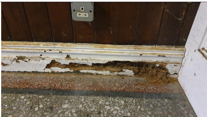
Figure 5 Evidence of timber decay – possibly dry-rot at junction with floor
