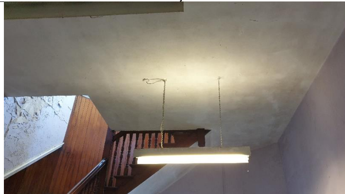
Figure 8 Lime Plaster ceiling with hair line cracks – no decorative moulding
