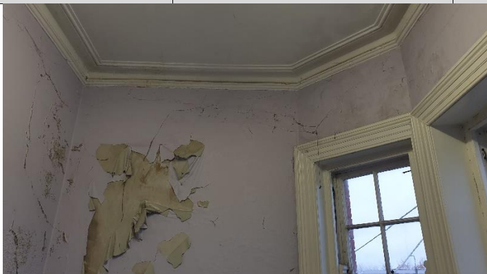
Figure 1 Boasted plaster at high level above half landing to stairs - Due to leak in roof above - extremely poor condition
