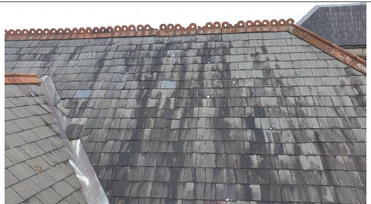
Figure 4- to right hand side of stairs out-crop Loose and broken slates at valley gutter at stairs out crop Damaged terracotta sections of ridge pieces
