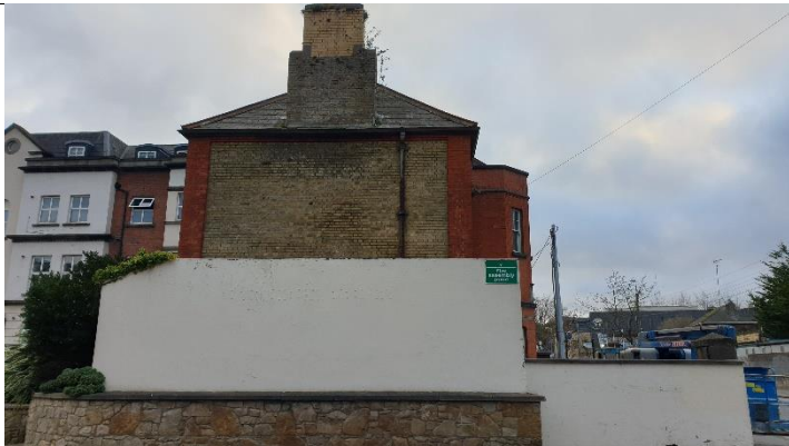
Figure 7 change of colour of brickwork to upper section suggests chimney has been rebuilt or extended
