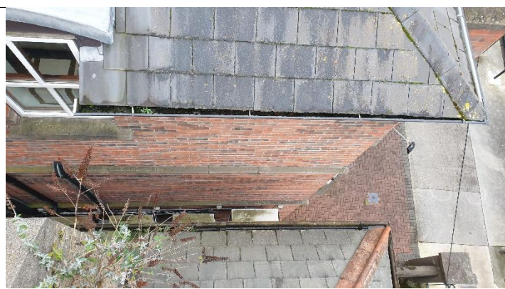
Figure 4 View of gap from above Narrow gap making maintenance of rainwater goods difficult.
