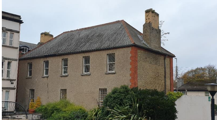
Figure 1 Lime "Harling" or roughcast render to east wall with brick quoins at corners.
