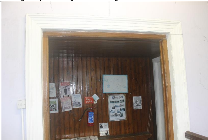
Figure 5 Large opening in wall where double doors had been previously
