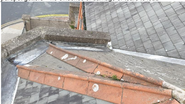
Figure 5 Terracotta hip tiles at junction of splayed section of roof Complex junction which h could be the source of water ingress
