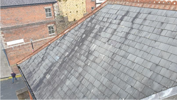
Figure 1- to left hand side of stairs out-crop Original natural slate roof with sections of recently slipped and previously repaired slate.
