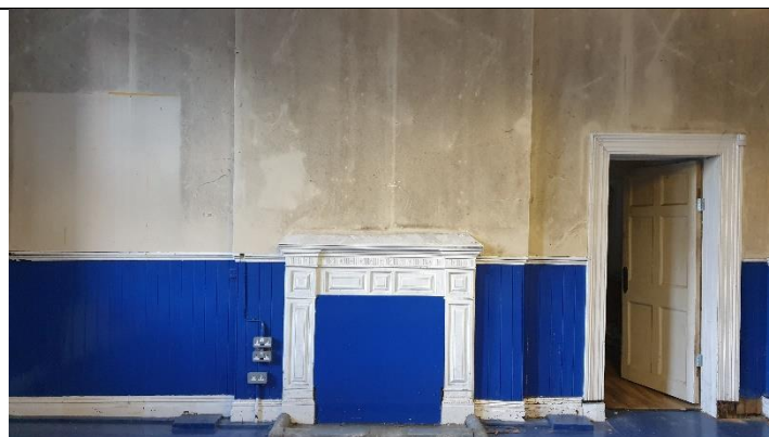
Figure 4 wall above fireplace is covered with plywood , suggesting poor condition of plaster work behind
