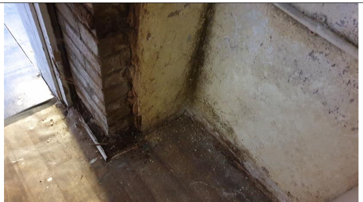
Figure 4 Boasted plaster at high level to RHS and LHS of window
