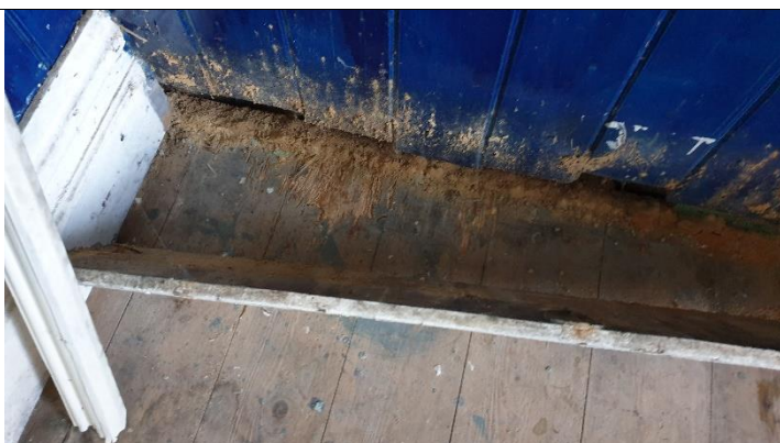
Figure 5 Yellow spores, suggesting dry-rot, evident along floor at edge of east wall, ground level to east is raised above internal floor level.
