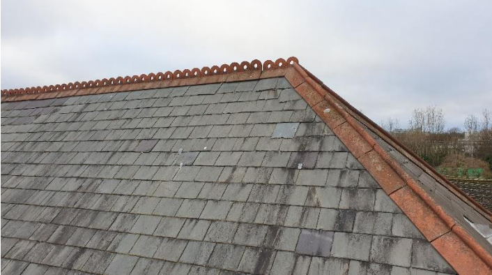
Figure 5 north-east slope with further examples of recently slipped and previously repaired slates using lead strap hangers - some evidence of recently replaced slates
