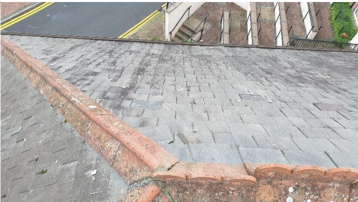
Figure 7- to left hand side of stairs out-crop Ridge pieces out of alignment and loose
