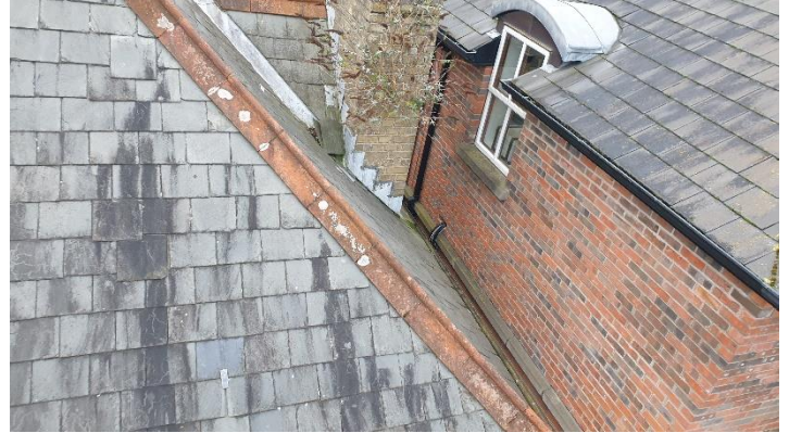
Figure 2 View of roof from the south -west Note slipped slates at gusset roof and buddleia
