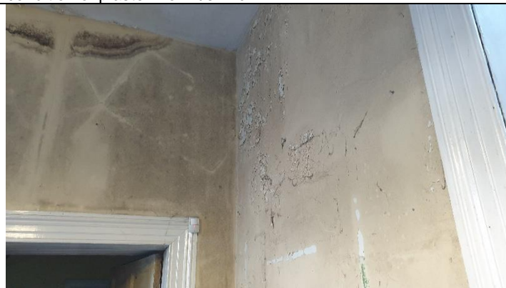
Figure 6 Boasted plaster at high level to LHS of window to Tea-station
