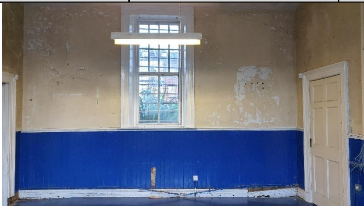
Figure 1 Evidence of timber decay along full length of walls to east – skirting detached from wall- walls damp
