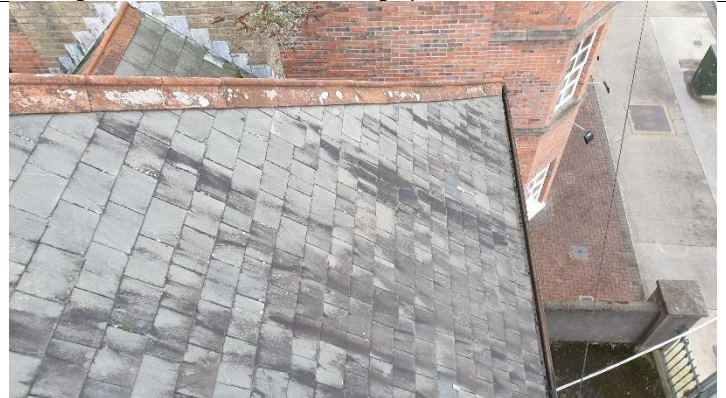
Figure 6 - to right hand side of stairs out-crop Section of roof in relatively good condition with less broken and slipped slates
