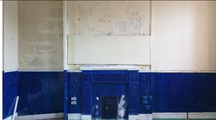
Figure 2 Severely boasted plaster at wall above fireplace, above dado rail.
