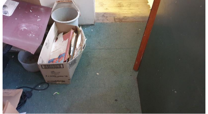
Figure 2 Vinyl sheeting to office in poor condition
