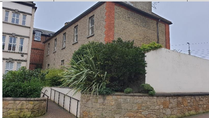
Figure 2 Significant changes in level at east face of building
