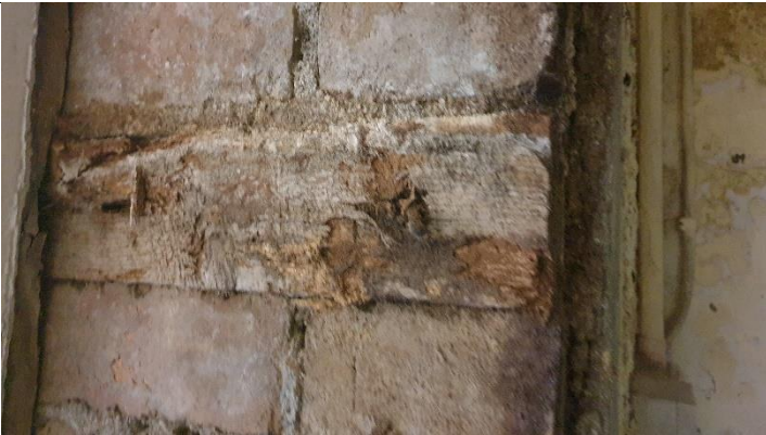
Figure 5 Evidence of rising damp from high ground level outside of wall - extremely poor condition
