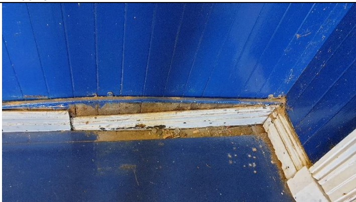
Figure 5 Floor sloping towards east– evidence of serious timber decay and possibly dry rot
