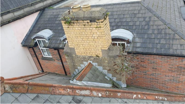
Figure 1 South face of roof with hipped slope, chimney at gable end with slated gusset roof connection to main roof.
