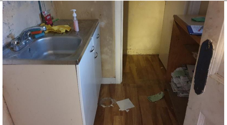
Figure 6 Counter to tea station - extremely poor condition
