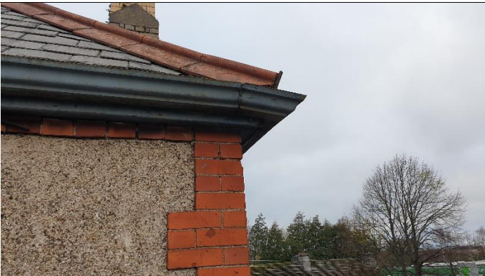
Figure 3 Gutter section at north-east corner sloping away
