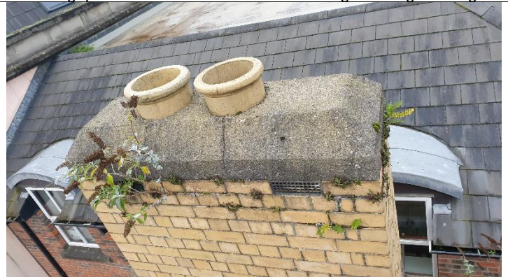
Figure 8 Cracks in concrete coping, pots appear to be flue liners Note vents in chimney stack
