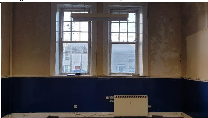
Figure 3 Hairline cracks in plaster at high level to walls to each side of windows
