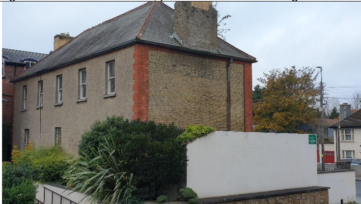
Figure 5 Buddleia above roof to out-house
