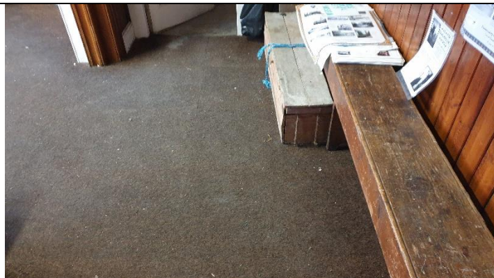
Figure 4 Carpet to lobby area in poor condition
