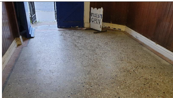
Figure 6 Terrazzo floor with some wear adjacent to the entrance door –
