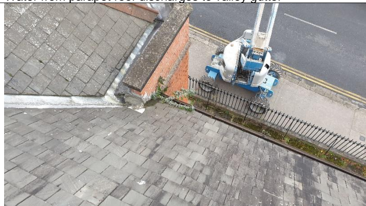
Figure 8 View of north west roof face from above Water from parapet roof discharges to valley gutter
