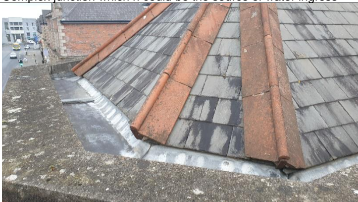
Figure 7 Wrought iron hip irons at end of terracotta hip tiles showing signs of rust
