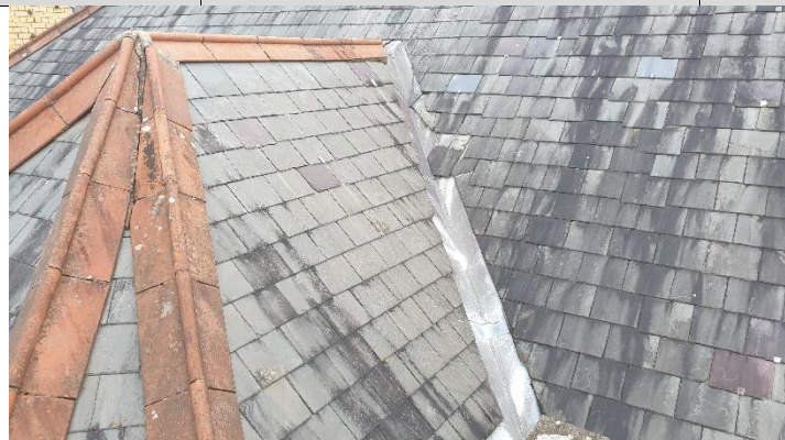
Figure 2- Loose and broken slates at valley gutter at stairs out crop This appears to be the source of the water ingress issues to the walls of the stairs
