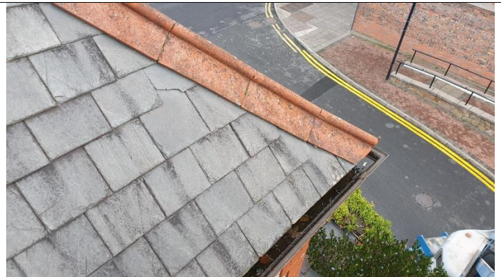
Figure 4 Corner broken slate next to terracotta hip tile
