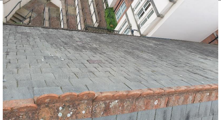
Figure 8 View of south-east slope of roof - showing slipped slates and terracotta ridge out of alignment
