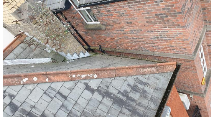
Figure 4 Cast iron gutters fixed to fascia at wall below in need of painting and rust protection
