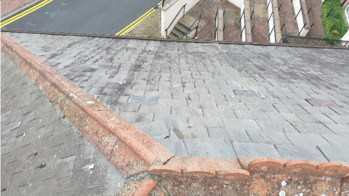
Figure 7 View of north-east slope of roof - showing slipped slates and terracotta ridge out of alignment
