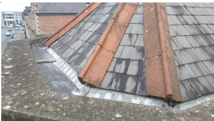
Figure 3 Close up of low parapet wall at stairs with lead flashings to parapet gutters – no evidence of damage or tears to lead
