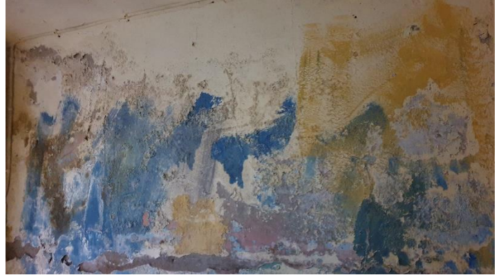
Figure 2 Severely boasted plaster at high level above counter - extremely poor condition
