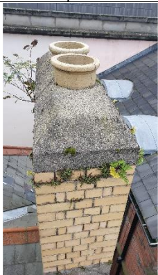
Figure 7 Mortar to brick work has been affected by weathering and is allowing buddleia to take hold and damaging brick work.
