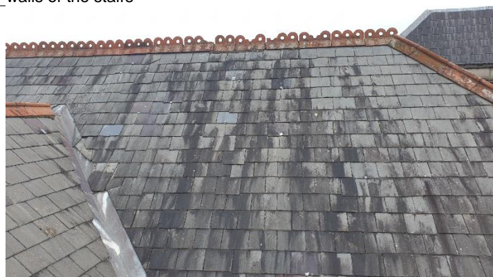
Figure 4 Further view of south west roof face with slipped and broken slates
