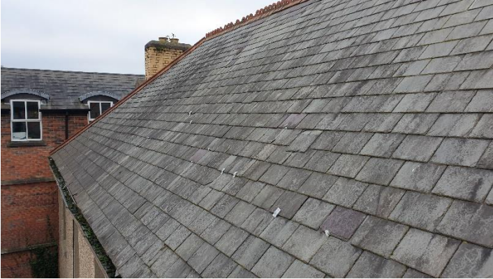
Figure 1 Original natural slate roof with sections of recently slipped and previously repaired slate.
