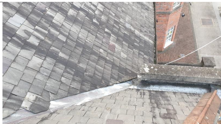
Figure 6 Further view of south west roof face from above Water from parapet roof discharges to valley gutter
