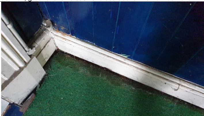
Figure 7 Evidence of serious timber decay and possibly dry rot – requires further investigation to establish extent
