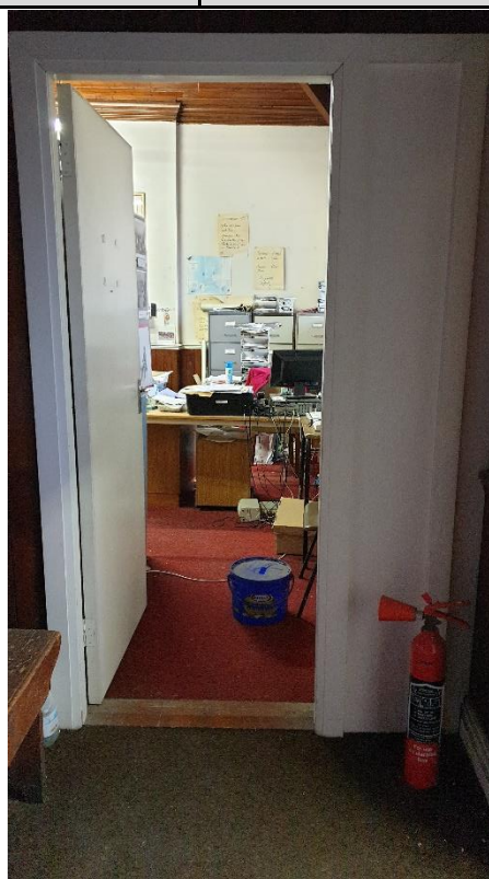
Figure 2 1 solid flush door – painted finish – door has not been upgraded and not considered a fire door
