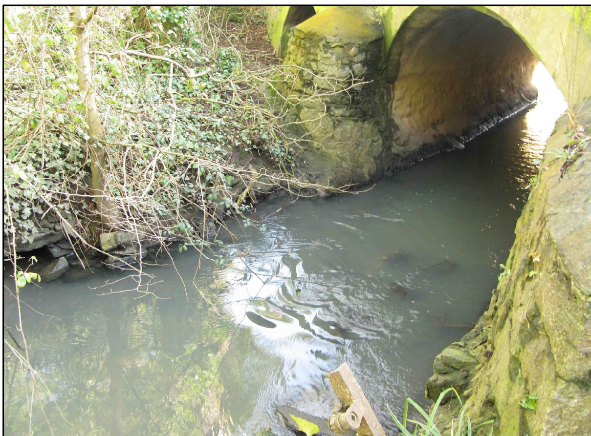
Plate 6: View of Pill River at kick sample site just upstream of road bridge.
