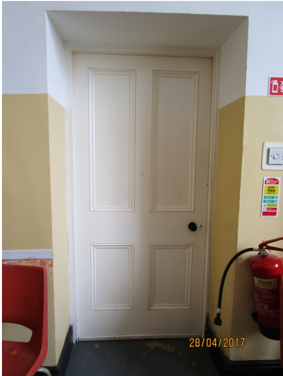
Plate 10. Typical four panel door within the building. It is proposed to retain these doors and make any necessary repairs .
