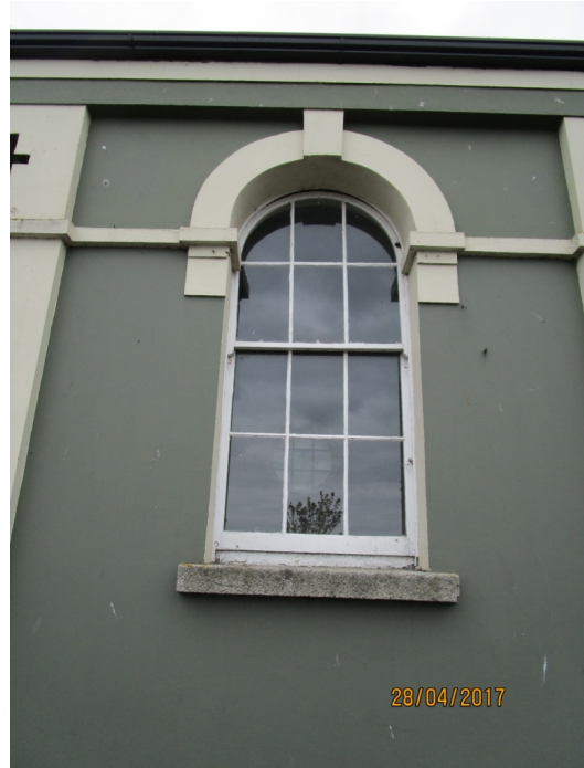
Plate 7. Window on North elevation. These timber sash windows will be repaired and re-decorated.
