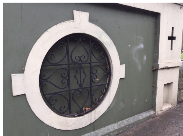
Plate 13. Circular window seen from exterior. This is one of two windows located at either end of the Southern elevation which is currently blocked up. It is proposed in these works to unblock the opening and reinstate a window to match the two central circular windows in detail.
