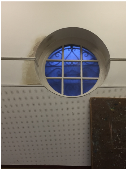
Plate 12. Circular window at high level in main hall. These windows will be repaired where necessary by a specialist sub-contractor and re-decorated.
