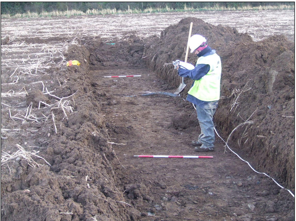
Plate 10 View E of BT9, showing enclosure (ditches demarcated by ranging rods) and disused modern water pipe (Field 12)
