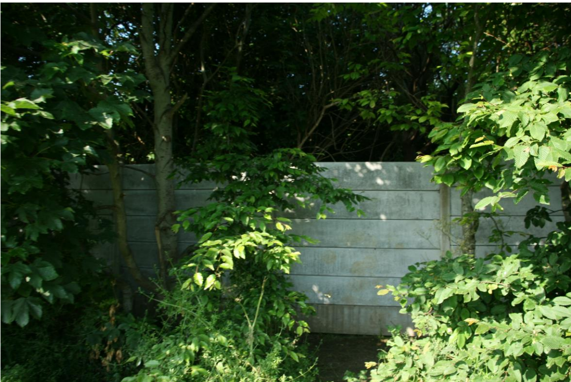
Figure 3: Photograph of the concrete post and panel fence along the southern boundary of the site.
