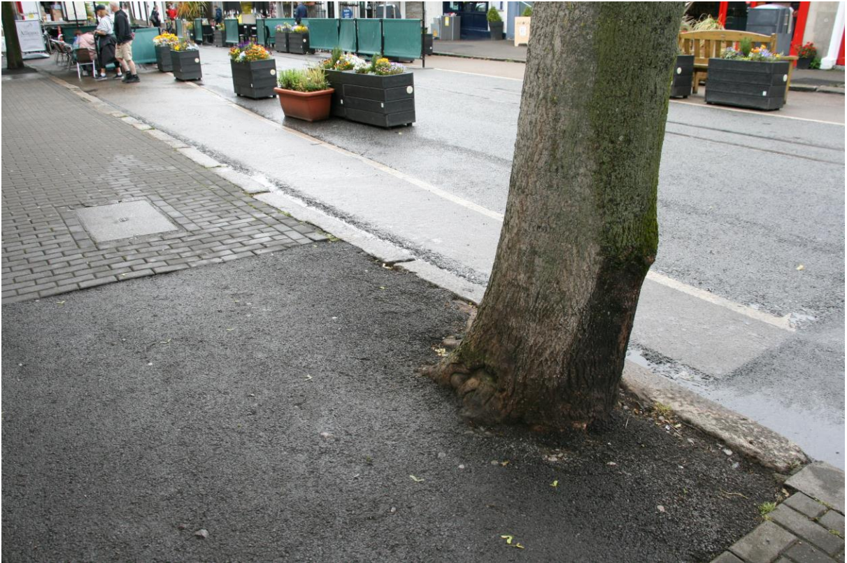
Existing trees at New Street. Black rubber surfacing has been installed locally to replace lifted and cracked paving.
