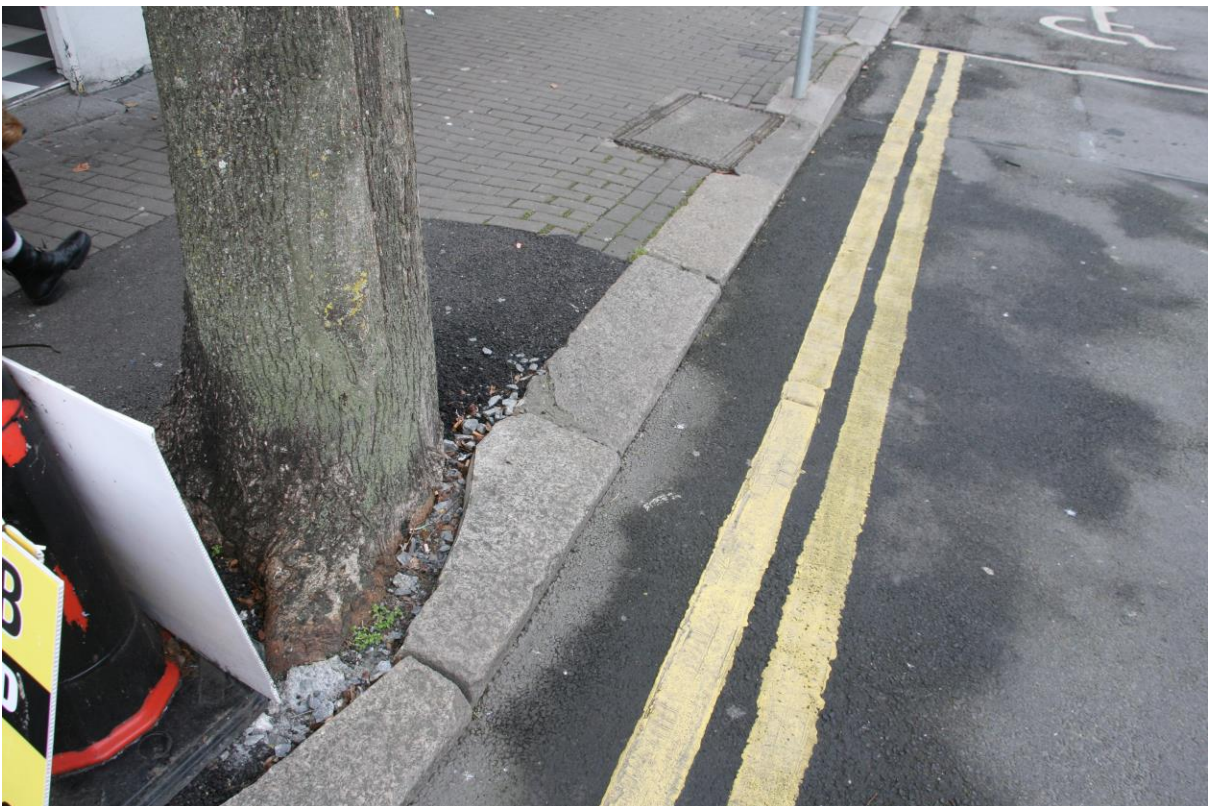
Existing trees at New Street. Granite kerbs are pushed out of alignment at the base of the tree.
