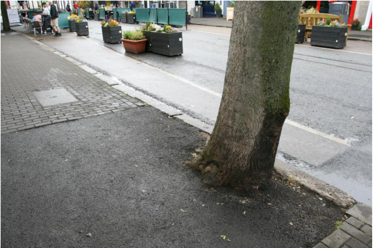
Existing trees at New Street. Black rubber surfacing has been installed locally to replace lifted and cracked paving.
