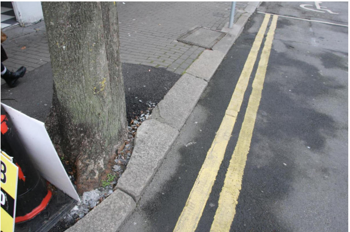
Existing trees at New Street. Granite kerbs are pushed out of alignment at the base of the tree.
