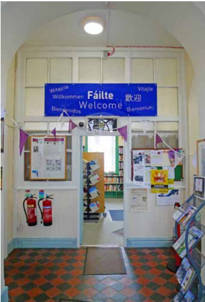
View of the hall looking in from the front door. The screen to the library is probably original. The jumble of signs, wires, etc should be removed.
