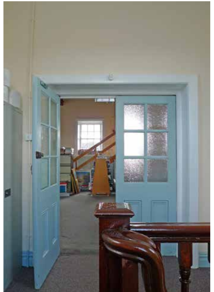
The same doors looking in towards the first floor library space. These doors are one of the finest features in the building and should be retained.
