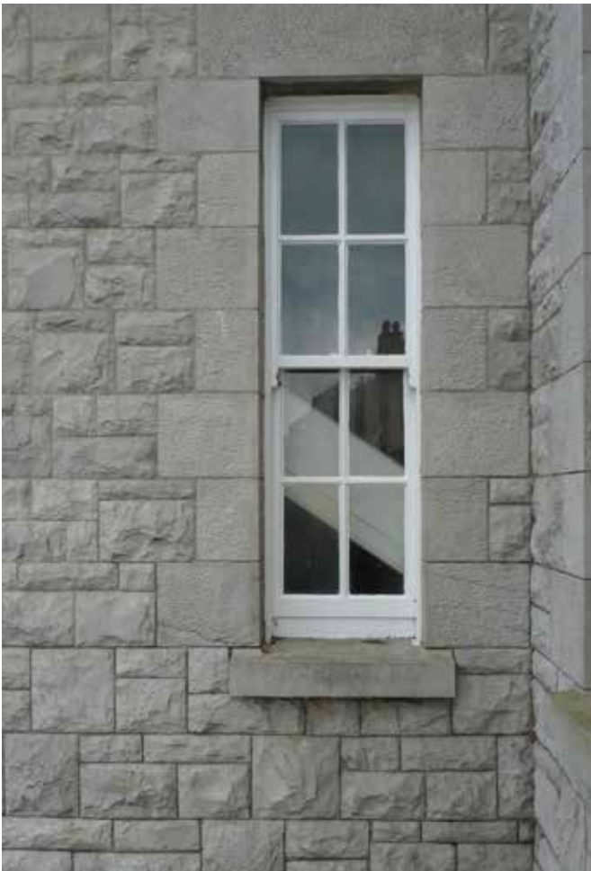
4 over 4 up and down sash window on the stair tower. Generally the windows appear to be in reasonably good order, but some paint is peeling
