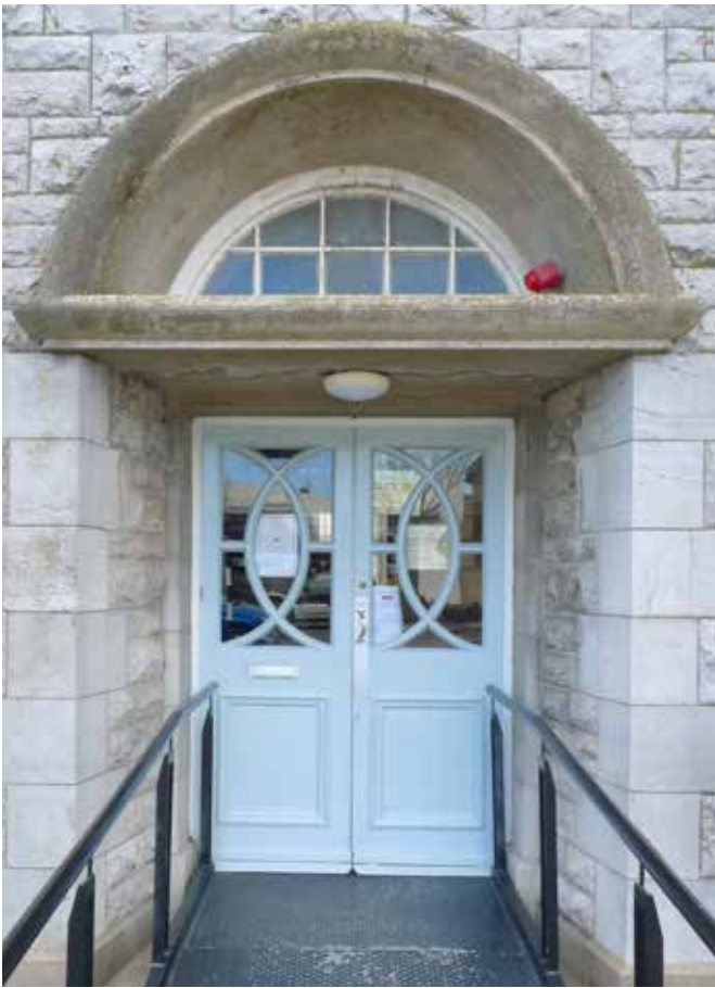
Entrance door the Skerries Library. The ramp and handrails for disabled access are very intrusive, as is the alarm sounder. The large casting over the door opening appears to have lasted well, but could do with careful cleaning. How it deals with water run off is uncertain
