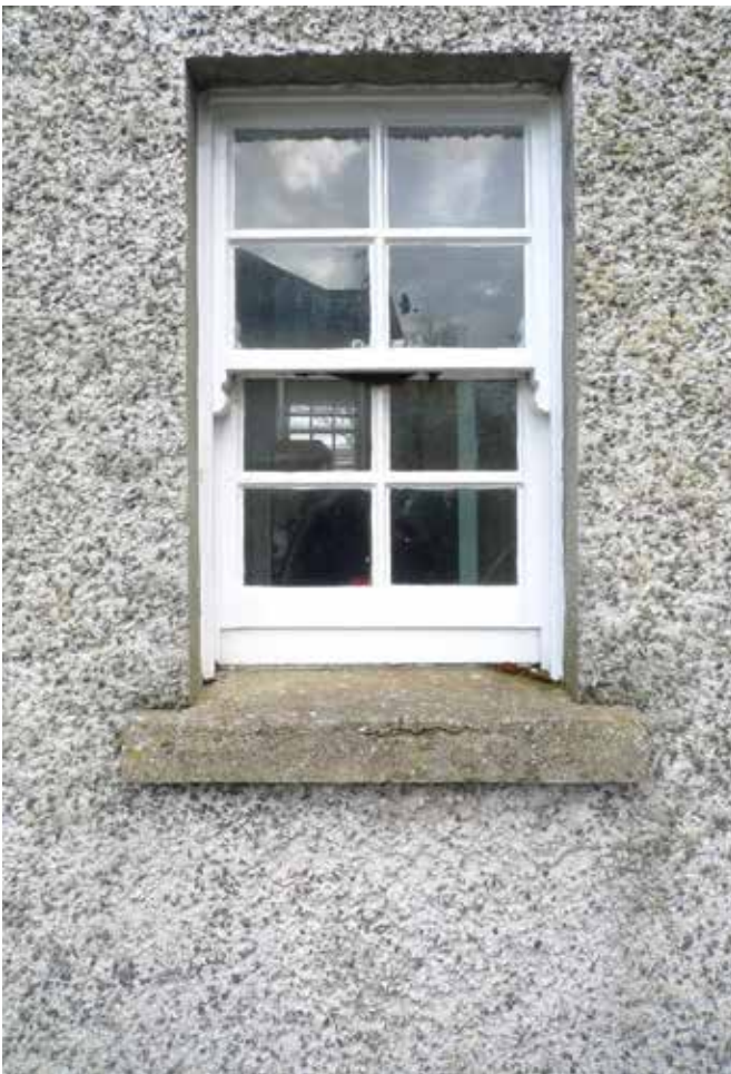
Small 4 over 4 up and down sash window in the small rear return. There is evidence of cracking in the sill
