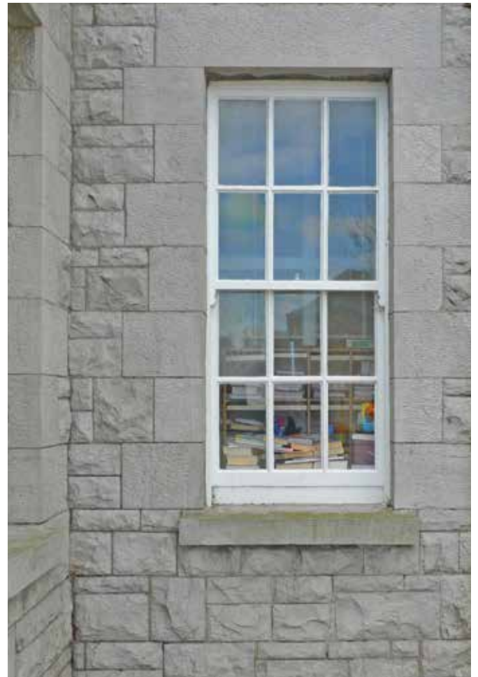
6 over 6 up and down sash window on the front facade. All windows should be checked and overhauled and repainted where necessary.
