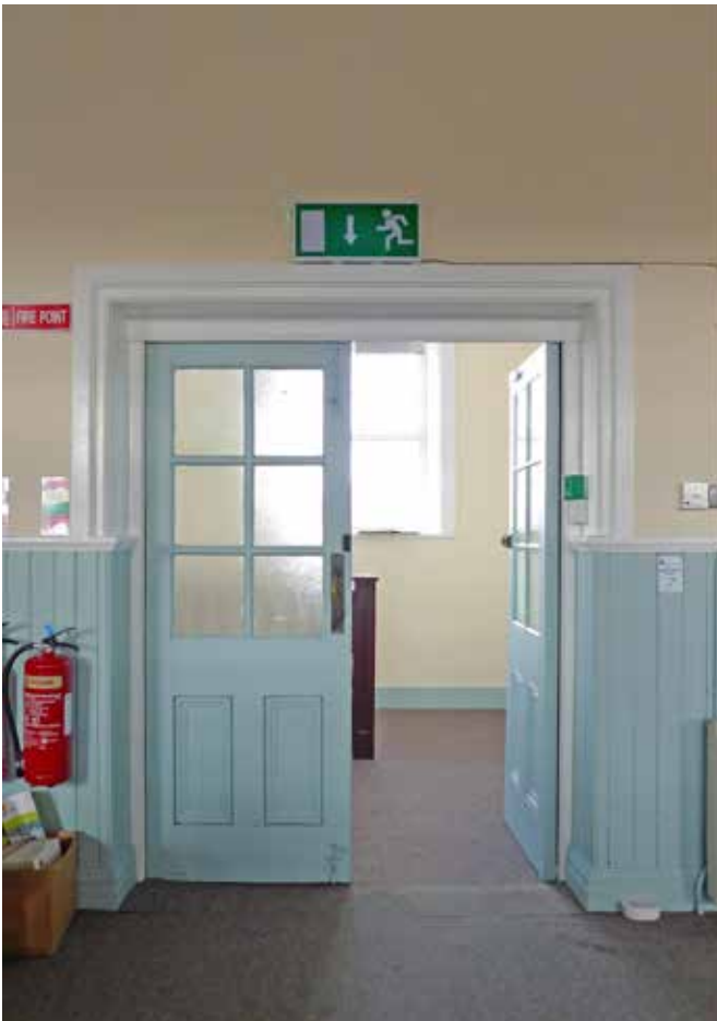
Double doors to the first floor library space, looking out towards the upper level of the stair hall. This pair of doors are very finely detailed, although they have been altered and some of the details do not match.
