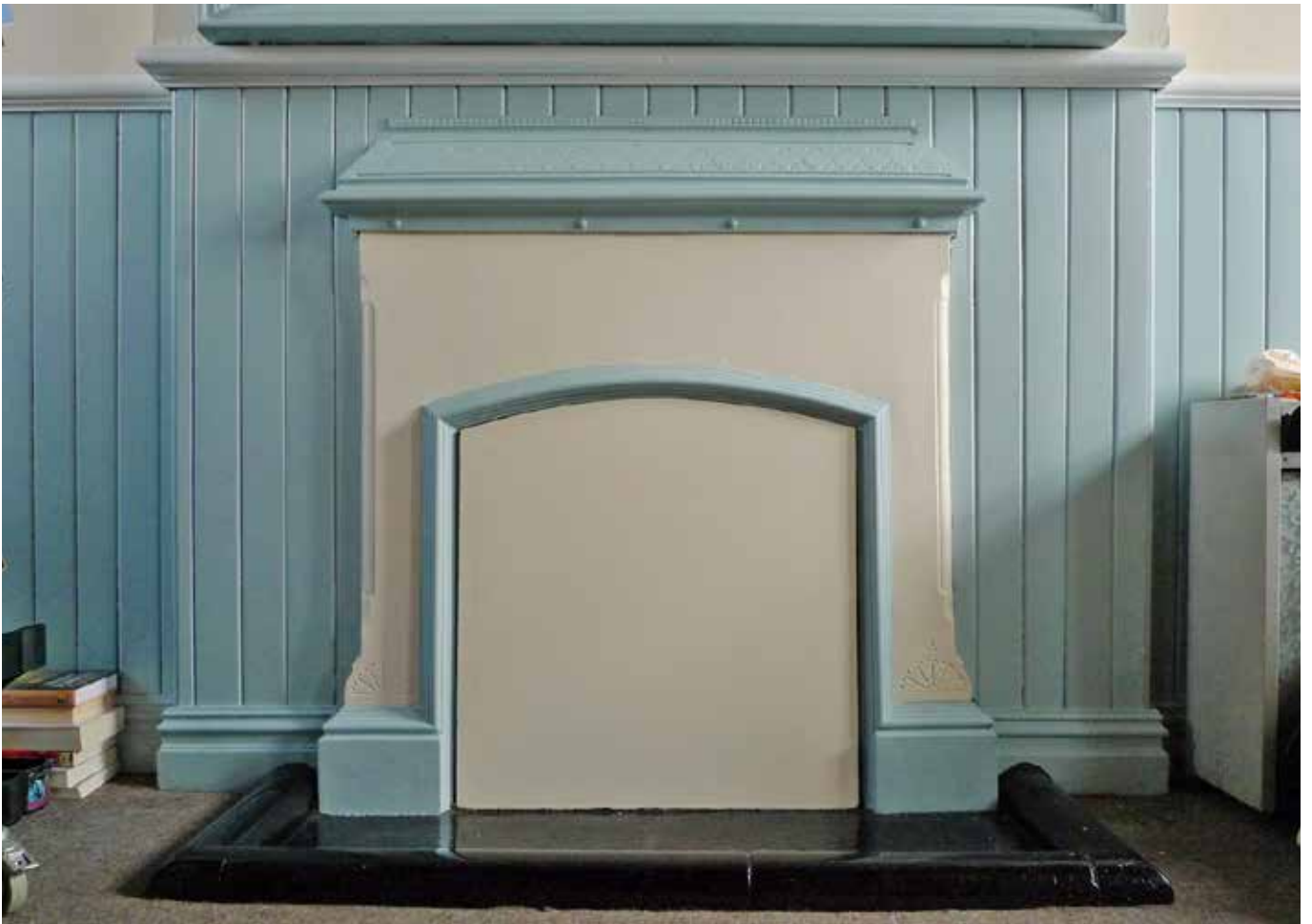
Cast iron chimney piece and what appears to be a painted stone hearth and surround, located at the south end of the first floor library space. These should be overhauled and perhaps have the paint removed. It appears that there were originally four such fireplaces.
